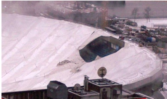
Collapse of B.C. Place Dome on Jan. 5, 2007
